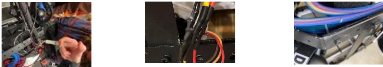
Figure 19: All exposed wires are waterproofed, covered with heat shrink and all sharp edges on frame removed.
