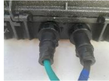
Figure 8: Tether connection to surface box
