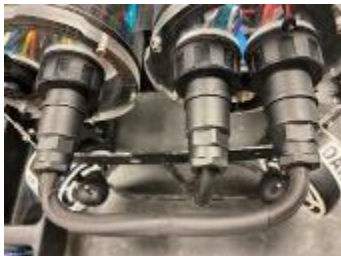
Figure 7: Bulgin PX 0747/8 power connectors between the two onboard control boxes.
