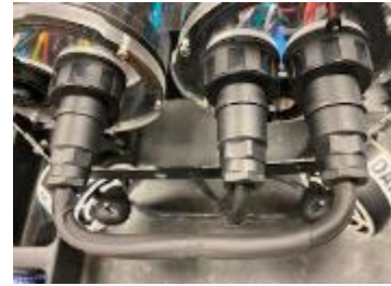
Figure 5: Bulgin connectors used for power distribution.
