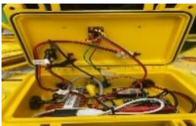
Figure 13:Control Box-photo by Araceli Orozco
