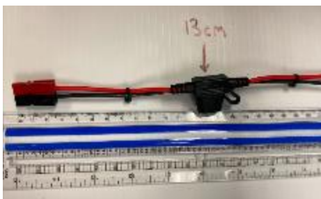
Figure 6: Fuse within 20 cm on main power line with Anderson Pole connectors
