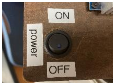
Figure 7: Emergency on/ off power switch located on surface control box.
