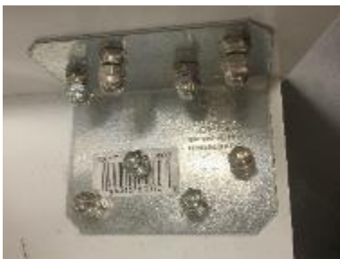
Figure 19: All sharp edges on frame was smoothed away, and caps were placed over fasteners.
