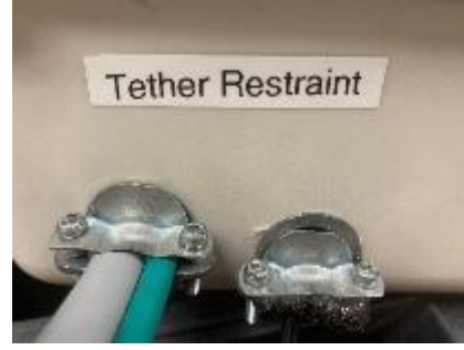
Figure 9: Tether restraints on surface control box.
