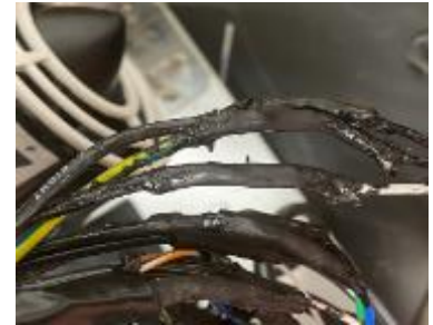
Figure 18: All exposed copper wire is waterproofed using heat shrink and liquid tape.
