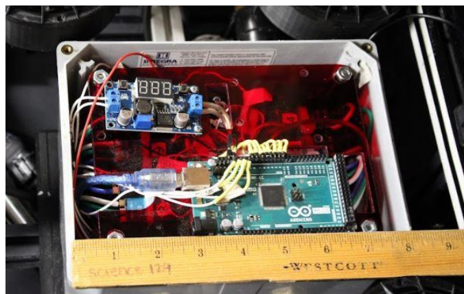
Figure 7: Wiring and Electronics inside of Dry Housing
