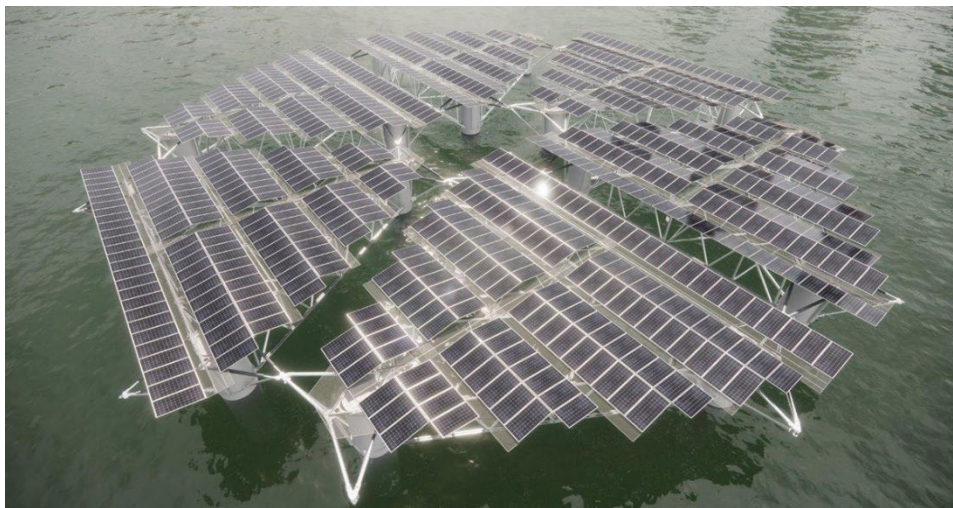
SolarDuck floating panel solar arrays ( SolarDuck and Partners to Build and Test Offshore Floating Solar Platform 'Merganser' | Energy | News (oceannews.com) )
