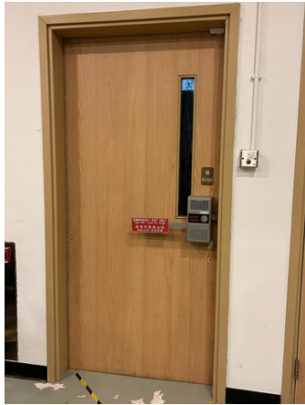
Figure 37: Fire rated door
