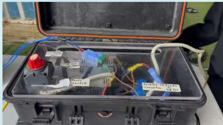
Figure 8: Topside power station featuring 48V DC conversion
