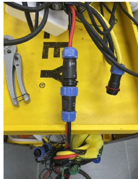
Fig3.8.3 Demonstration of Aviation Plugs Connected
