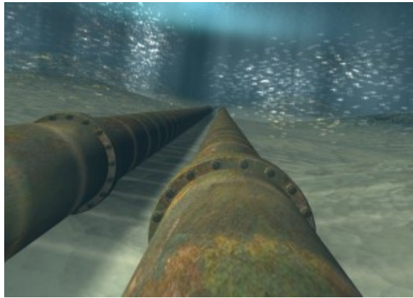
Corroded subsea pipeline ( http://subseaworldnews.com/2014/04/01/baosteel-yantai-delivers-subsea-steel-pipes-for-bohai-oilfield/ )
