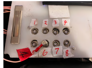
Figure 11 Signal reception ports on Control box
