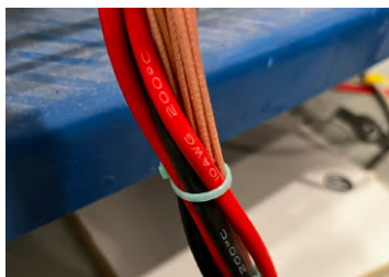
Figure 23.1 cables secured by zip tie
