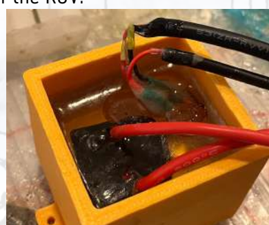
Figure 2.9 : picture of PCB covered in epoxy
