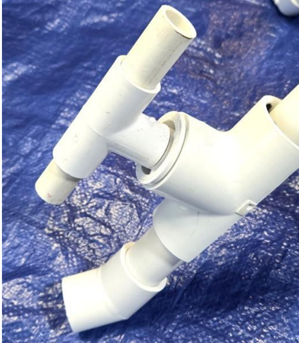
The epoxy patch applied over the corrosion on the base of the wind farm.
