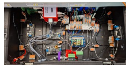
Topside Control Box Credit: N Scott
