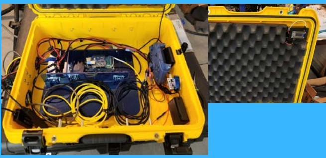
Figure 6: Control Box (without top covering panel).
