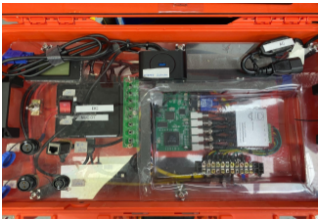
Fig.9 Interior of the topside control unit
