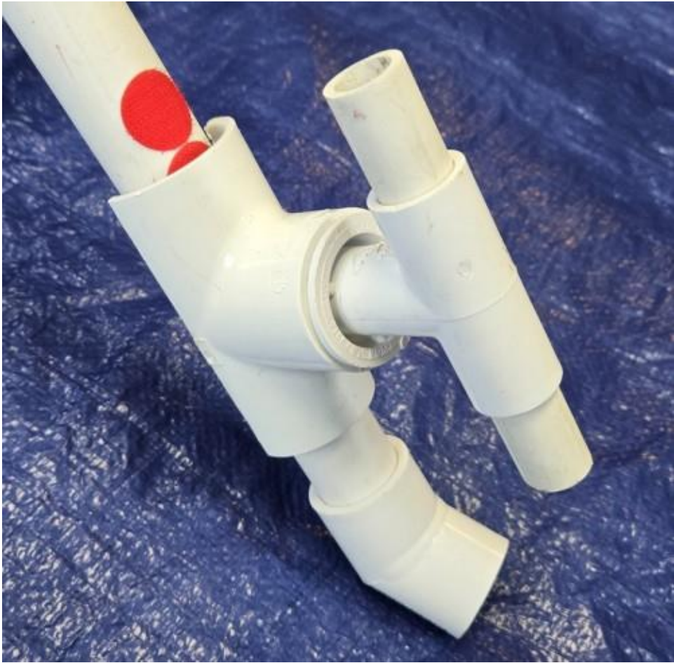
The epoxy patch applied over the corrosion on the base of the wind farm.
