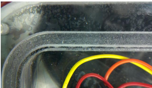
Figure 20: Failed O-ring Seal
