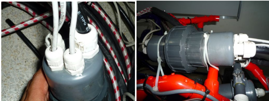
Figure 21. Left, plastic nylon cable gland PG9 (UTP cables) and PG 16 (No.10 AWG cable). Right, decoupling system positioned in the ROV tale. R.M.
