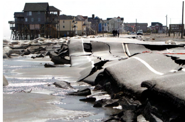
Figure 15: Damage done to local roadway (Photo: Rocky Mount Tribune)
