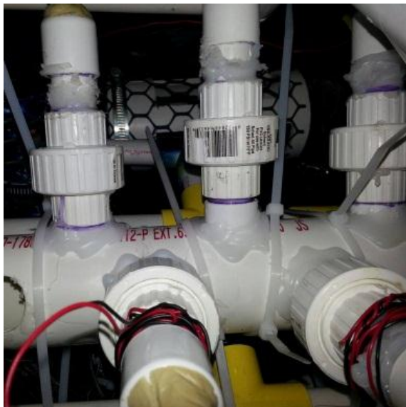
(Photo 9 – Small PVC Union “quick connects” configured in the V shaped manifold)
