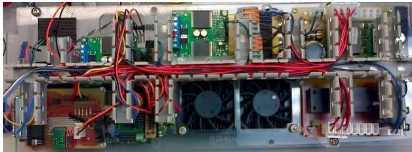
Figure 9: Electronics enclosure showing layout and wiring
