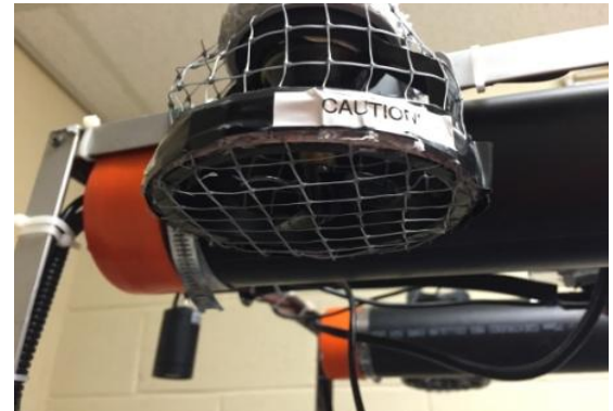
Figure 30: Protective covering around motors. (Credit: Maria Halleran)
