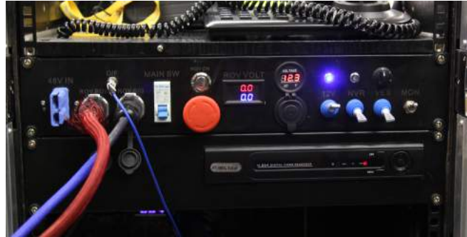
Figure 40: EDCP showing the ammeter and voltmeter for troubleshooting
