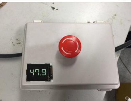
Figure 38 Emergency kill box with voltage reading from a digital screen
