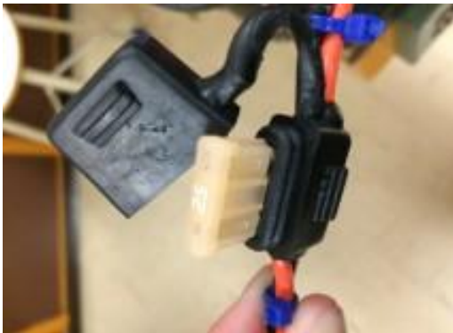
Figure 26: A 25A fuse inside fuse holder on positive lead. (Credit: Daniel Drodge)
