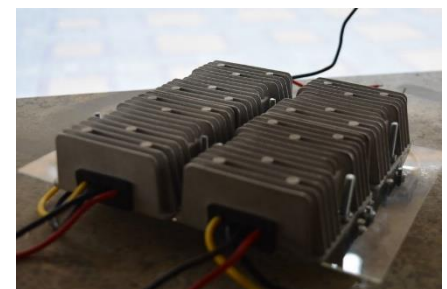
Figure 28. Four DC-DC converters tied together on one of the electric box plates.
