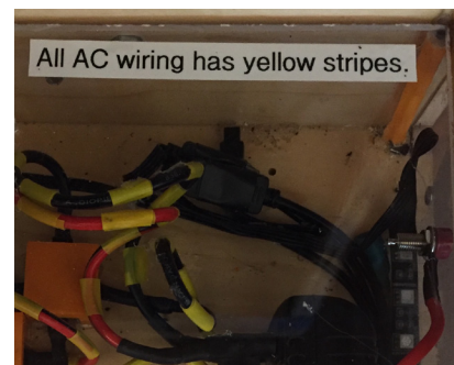
Fig. 19: The clearly labeled AC wiring in the control box.
