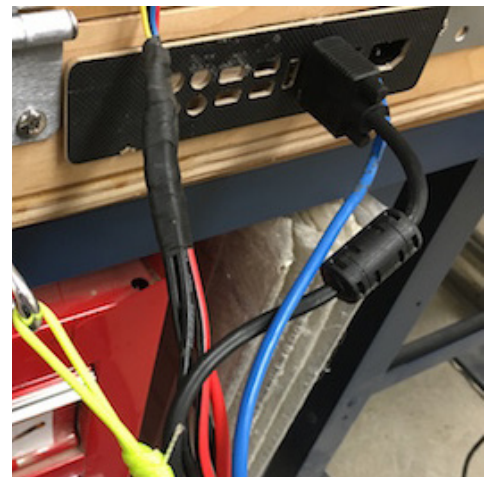
Fig. 12: The attachment point of the tether to the control box, showing strain relief.
