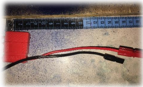
Photo #2: Distance between Anderson Powerpole connectors and fuse
