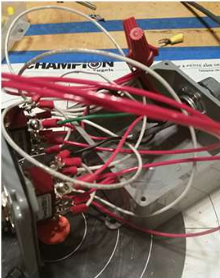
The inside wiring of one of the control boxes.
