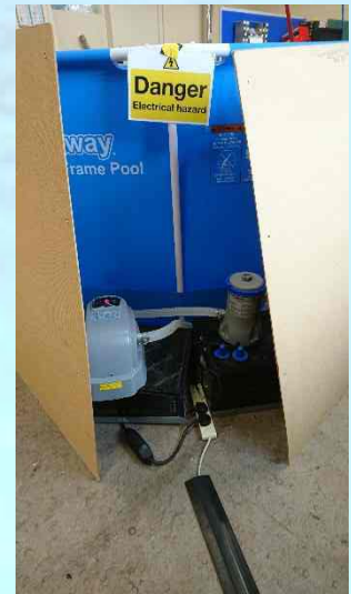
Fig. 34: Electrical Safety at Poolside
