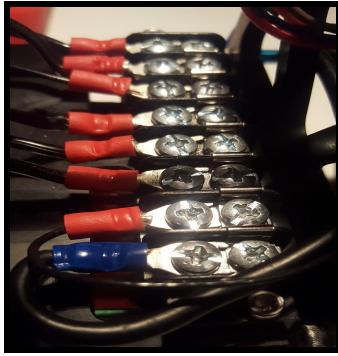
Figure 13: Power Distribution Block (Photo Credit: A. Fouad)
