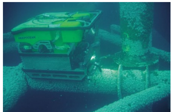
An ROV performing safety inspections similar to the Argo VI 's dam inspections (Photo Credit DeepOcean).
