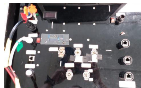
Fig 3.13a Main ROV Control panel
