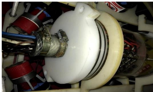
(Fig. 12: Control box sealing)
