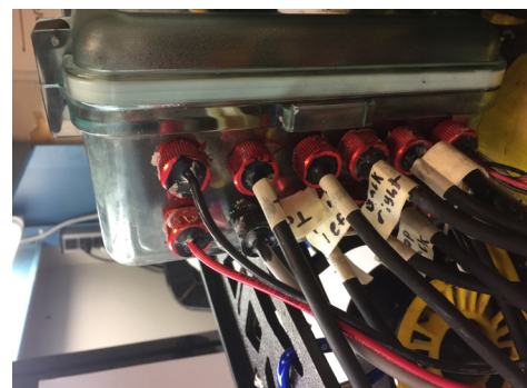
Fig. 17: Cable penetrators exiting the electronics enclosure
