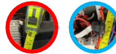
Figure 30: The power connector is fully built according to the requirements. (Image by Candy LEE)
