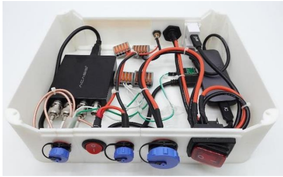
Figure 20 Inside of Control Box
