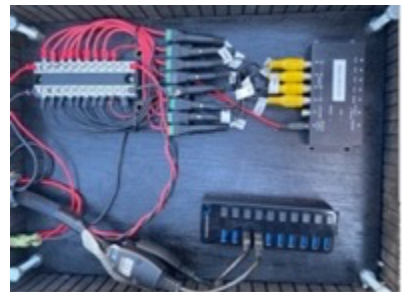
Figure 9: Surface control box
