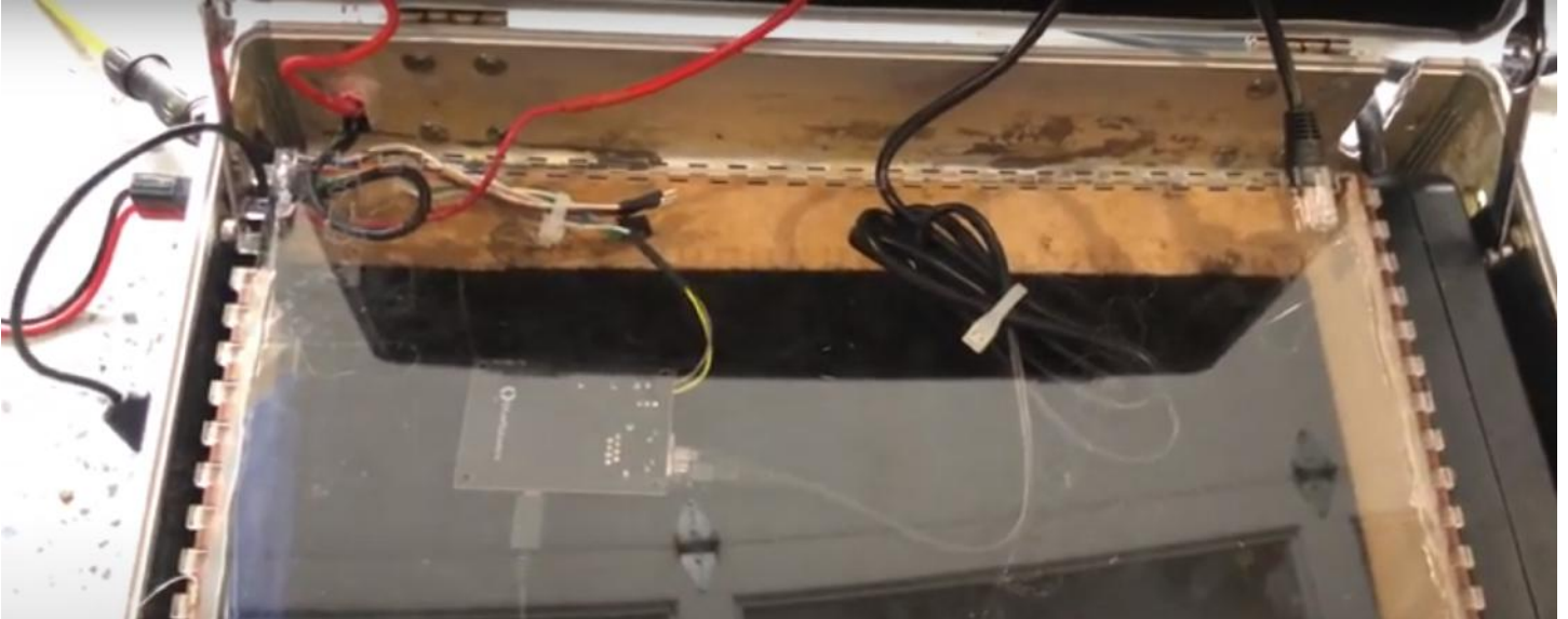
All wiring in the control box with the laptop removed (Image by Kavi Dey)
