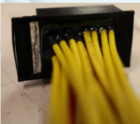
Figure 11. Power Distribution Board
